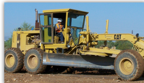
140G Blade prepping fill areas on a site at DC Ranch in the early days.
